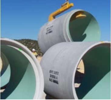
SRC pipes with corrosion protection 29
