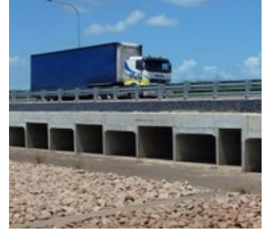
Box culverts - large 51
